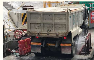
Automatically wheel washing system is set up at entrance and dump trucks are fully covered
